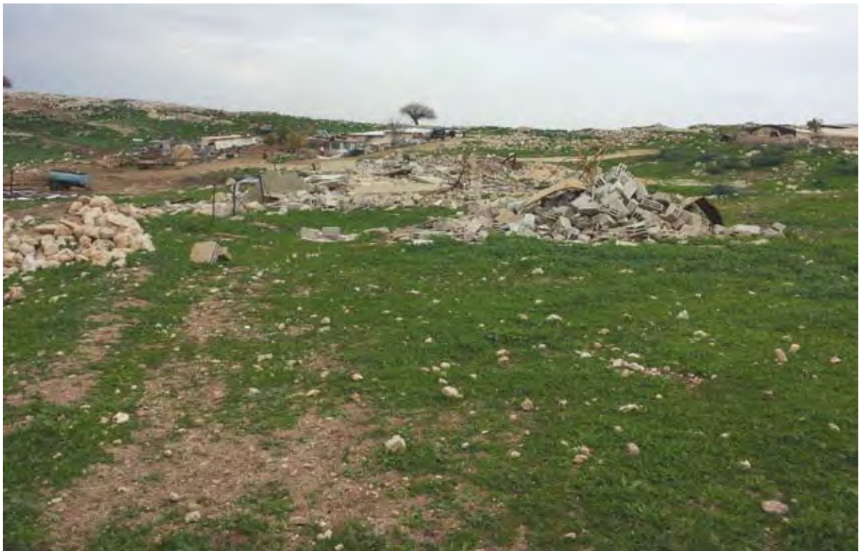
Demolished structures in Khirbet Yarza in Firing Zone 901.
